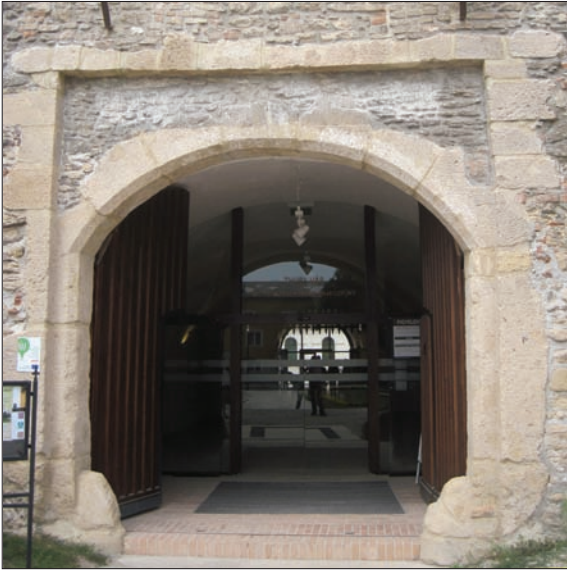
Fig. 7. Gate of the southern gate house with traces of the draw bridge (Várpalota Castle).
