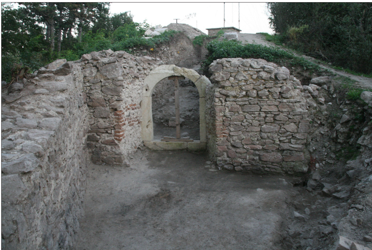
Fig. 3. The southern wall and the entrance of the tower (Photo: Dóra Hegyi).
